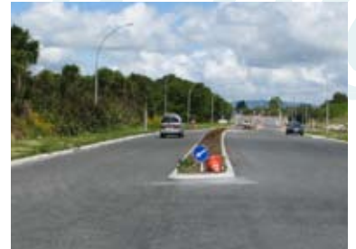
Wairere Drive looking west from Raungawari Drive. The final asphalt surface will be completed in April 2009.
