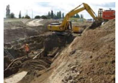
Pipe laying of the Far Eastern Interceptor 1050mm diameter sewer line at the eastern end of the site near Crosby Road.
