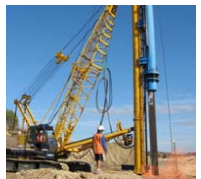
A piling rig driving steel piles in an in-filled gully. The piles are needed to support the weight of the FEI sewer line over the weaker ground as a measure to reduce the risk of settlement on the pipeline.
